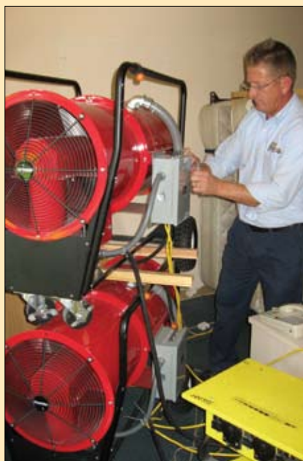
Massey Services' Tom Jarzynka prepares to power up the dual electric heaters used in the study.
